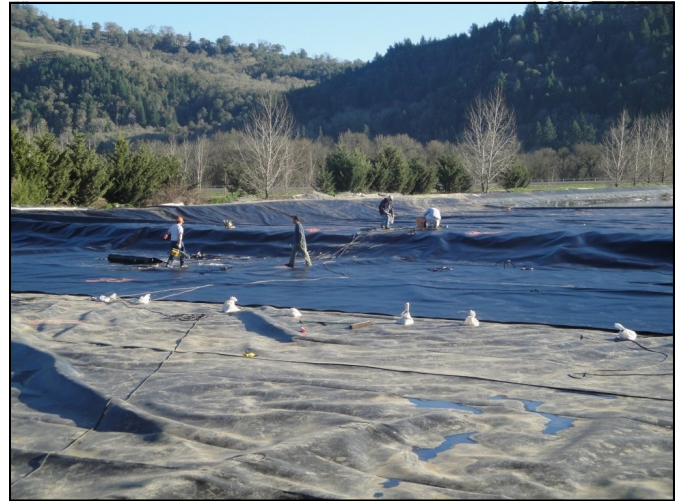
Workers from Industrial Environmental Concepts, Inc. of Minnesota spent several weeks in Roseburg installing the lagoon covers. They helped stimulate the local economy with lodging and food expenditures. Two of the workers also purchased used vehicles from Roseburg dealers during their stay.
