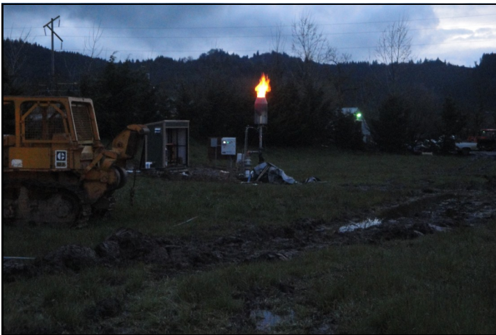
The floating cover traps the gases released as the waste degrades. The gas is then removed, monitored and burned through a torch flaring system. The system burns 24/7 and is visible from the I-5 freeway just north of Roseburg in the evening.
