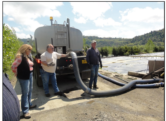
The City of Sutherlin trucks in its septage to Heard Farms for further processing and composting. From left, Tracy Loomis, consultant for the project, City of Sutherlin employee and a Heard Farm employee watch as the septage is transferred to the lagoon. Approximately 950,000 gallons of material are added to the pond on a monthly basis.
