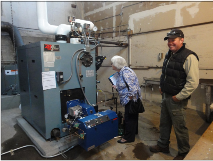
Oregon Department of Energy Project Manager Shanda Shribbs inspects Butte Falls' new energy-efficient boiler with Butte Falls Maintenance Director Jeff Gorman. The boiler was paid for with Recovery Act (stimulus) funds.
