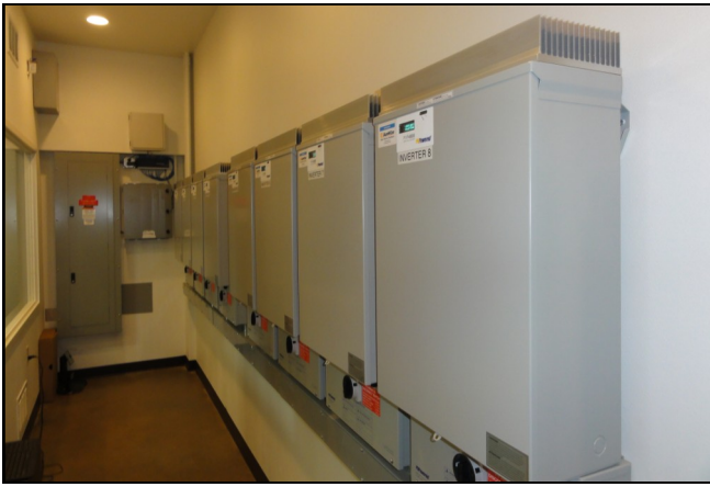
Fourteen inverters from Bend-based PV-Powered convert the direct electricity into alternating current for the Consumers Power utility grid.
