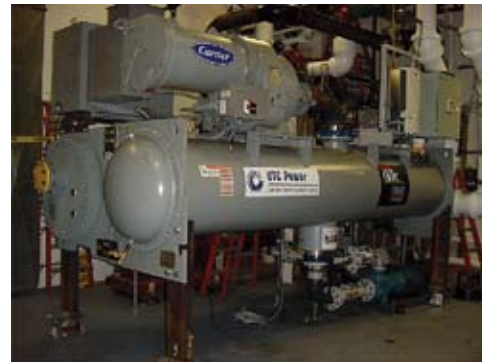
PureCycle® Geothermal Power System installation in Chena, Alaska
