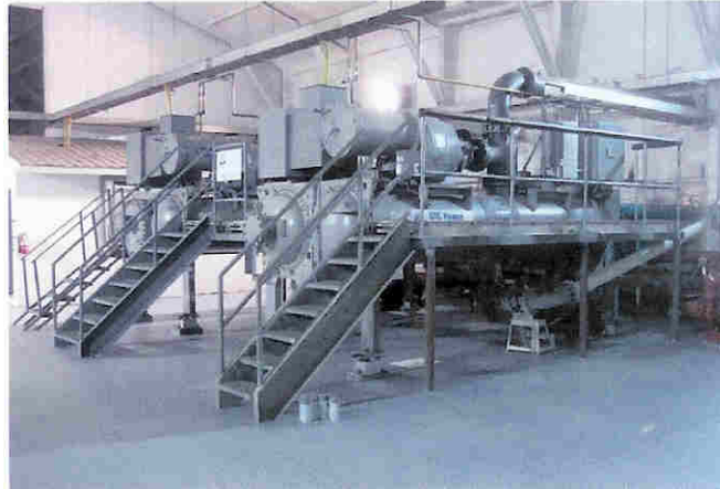
Figure 1 Two 250 kW United Technologies ORC units located at Chena Hot Springs Alaska
